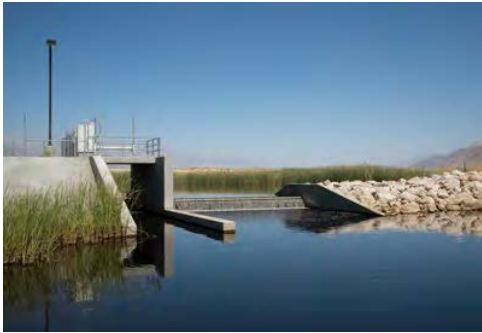
17. Main LADWP Pump Back Station, Owens Lake, CA
